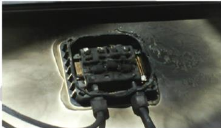
Burnt junction box
