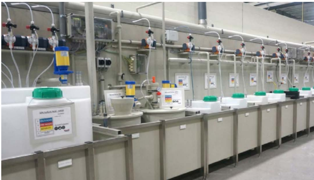
FIGURE 5 – Examples of automated chemical dosing systems.
