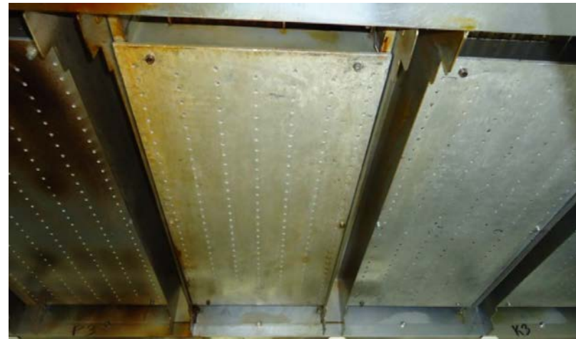
With slot exhaust and catalyst in first cool zone after 8100 boards
